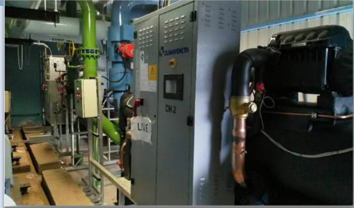
Commissioning of new Chiller plant using Skyspark for M&V
